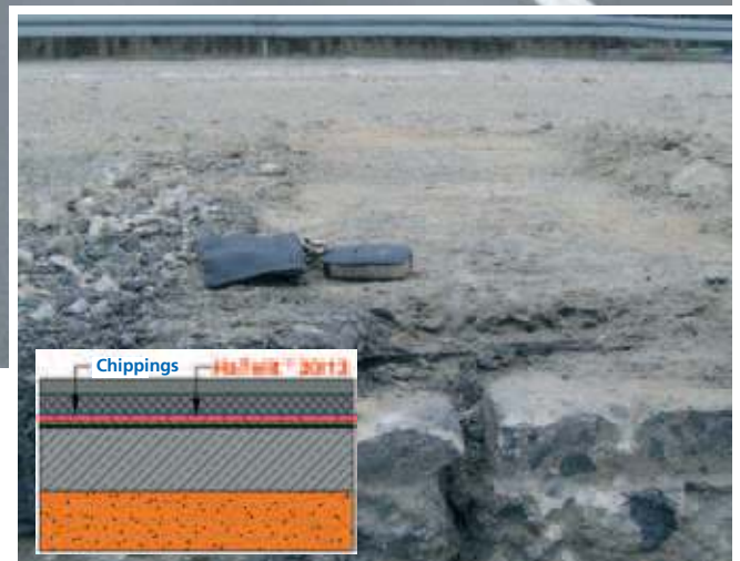
Part of German Highway 13 broken out during reconstruction in 2005 – remaining asphalt binder course above HaTelit® – no visible cracks
