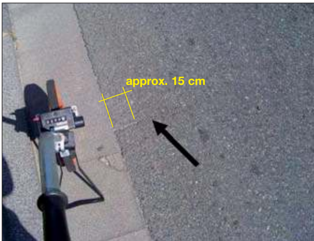
Cracks found in edge area, August 2009
