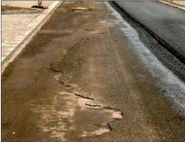
Condition of Rosenstrasse before overlay, May 1996
